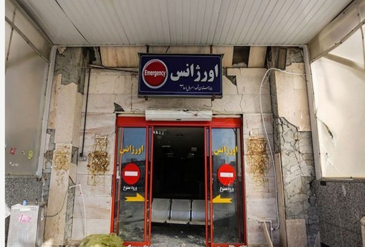
A dilapidated Emergency room in Sar Pol-e Zahab
